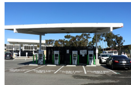
Solar Integrated Fast Chargers
