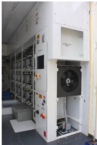
Demonstration Iron Flow Energy Storage System
