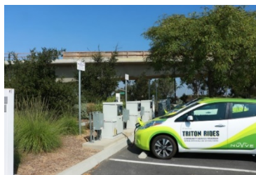
EV Charging Infrastructure
