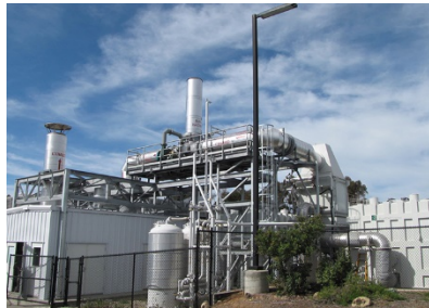
2.8 MW Fuel Cell
